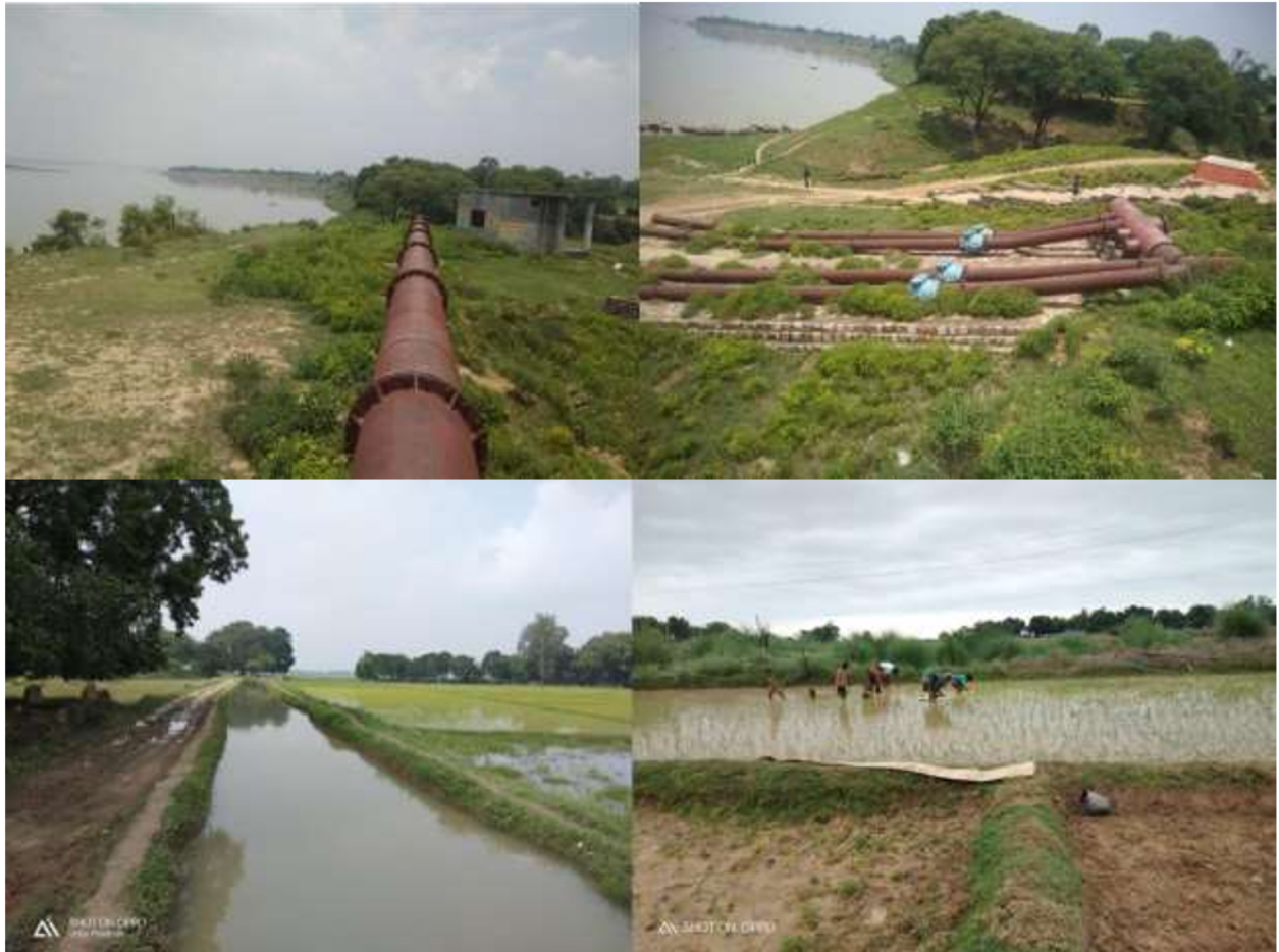
Plate 3.1 Water extraction from sanctuary area
